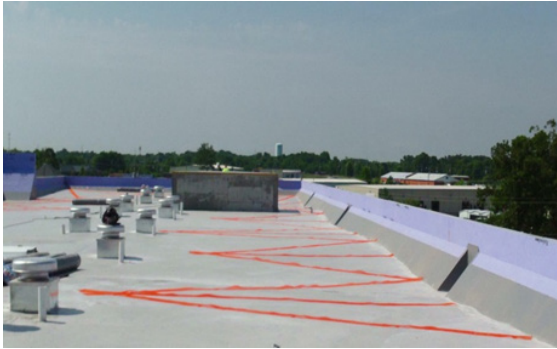
Distribution Strips Connect the Roof Perimeter to the VacuSeal Roof Vent
